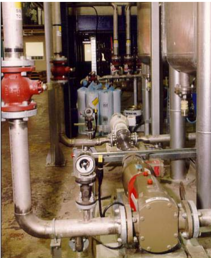
Series D4 pump handling UV resin with Series S3 pump handling water-base ink in background at printing ink plant in UK
