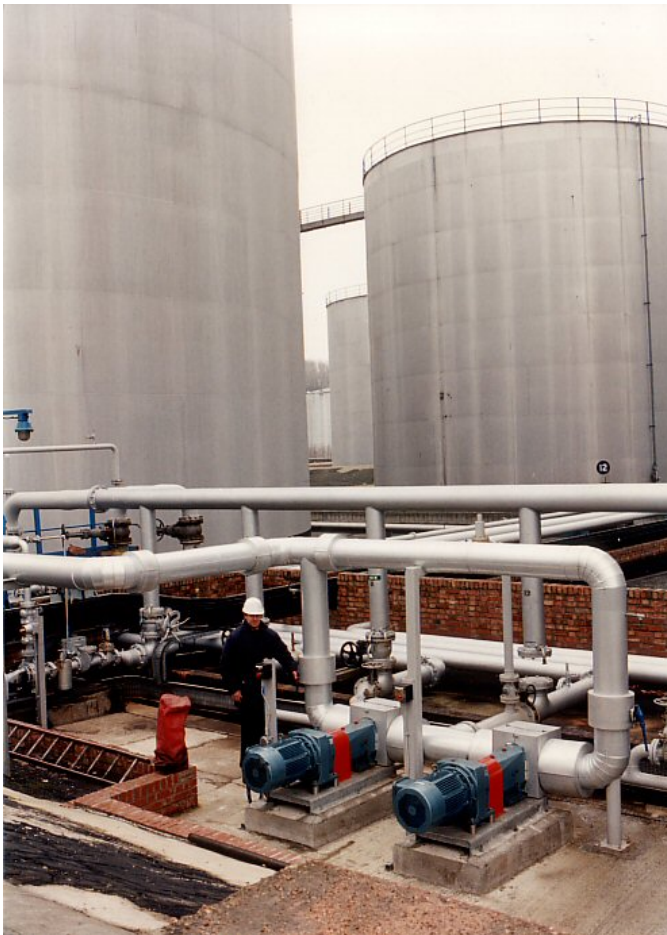
Series D6 pump at UK oil terminal used to feed a separator to remove hydrocarbon residues from surface water
